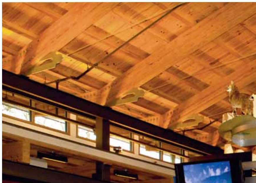
Dimming ballasts allow the concealed uplights to respond to available daylight.
