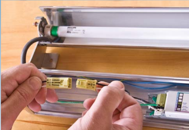
2-wire fluorescent ballast disconnect
